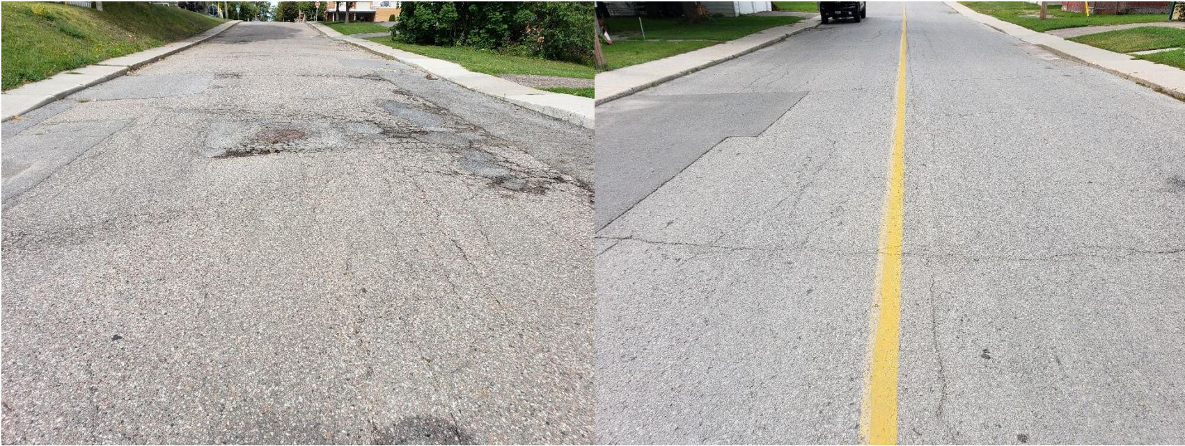
Sample Serious/Failed Road (0-25) (Grey & Dark Red)
