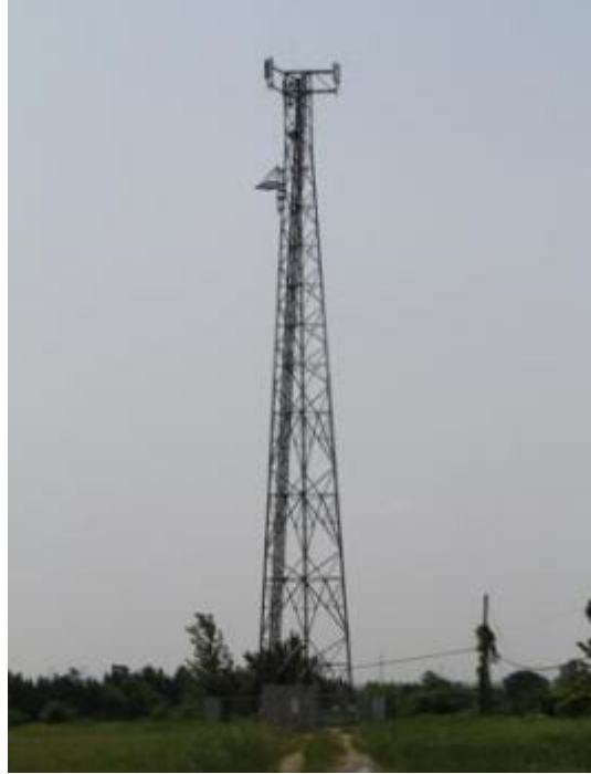
Figure 2- Example of Self Support Tower (Type S)
